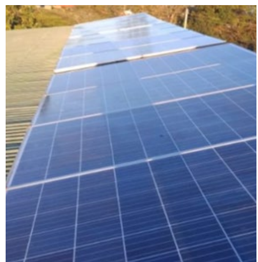
Sustainable off-grid community energy in Dedza District
