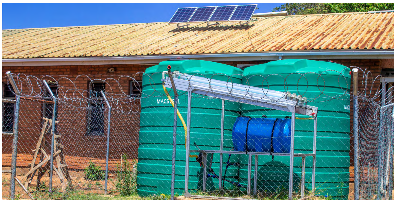
The Solar Water Disinfection Equipment set up at Thekerani Health Centre in Thyolo
